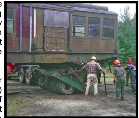
CC (red hardhat), helping to problem-solve getting a new arrival off the trailer it arrived on and onto track.
