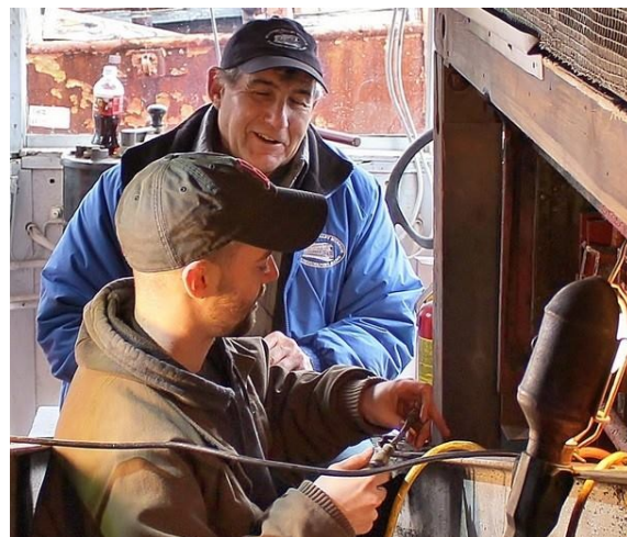
Dan Vardaro and Corey Reynolds service 5106's KM controller.
