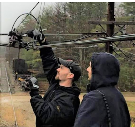
Header: Before construction begins, Fairview barn is getting switched out in preparation for the project. BB Above: Corey Reynolds and Brandon Barlow make an overhead repair to allow access to North Riverside yard. JP
